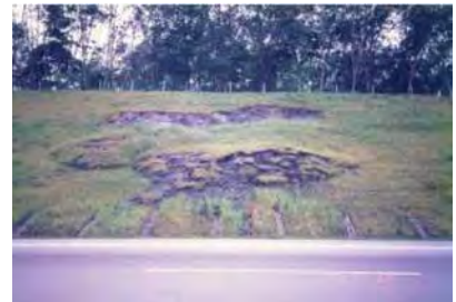
Figure 3: Slope failure in graphitic schist soils, Air Keroh.
