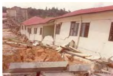
Figure 5: Slope failure due to rapid draw-down.
