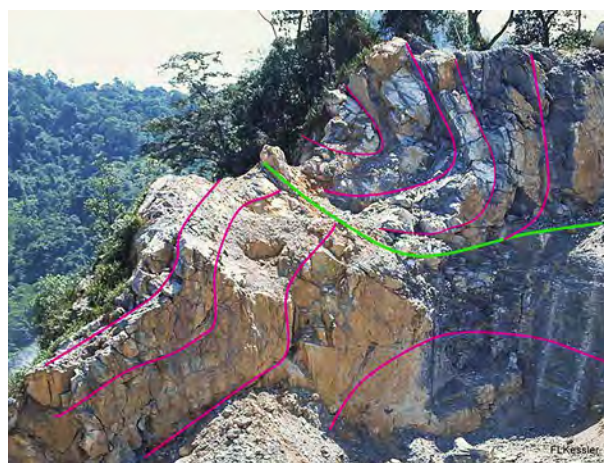
Figure 5: Cylindrically folded limestone section in the upper part of the quarry. This part of the quarry is loose with overhanging rock walls and forms an HSE risk.
