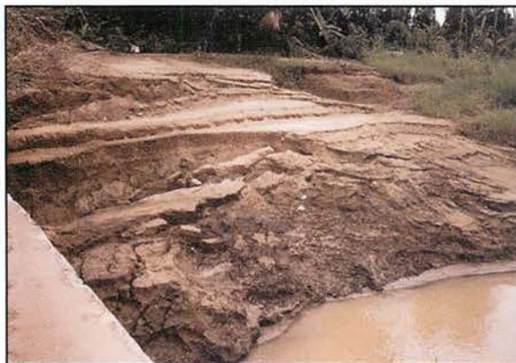
Fig. 11. Riverbank instability, Sarawak.
