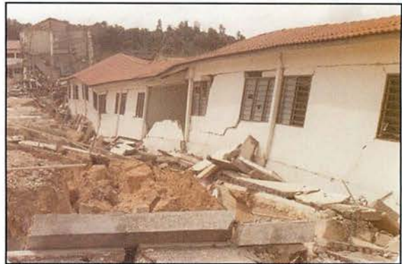
Fig. 12. Rapid draw-down of mining pond triggering slope failure and destroying houses, Kuala Lumpur.
