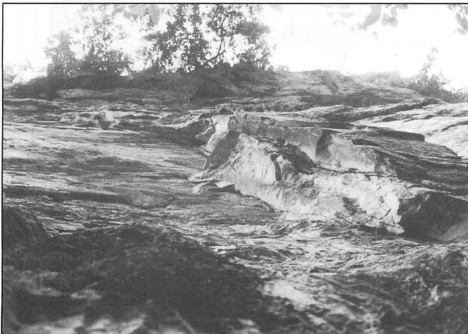
Figure 1. Slab/plane failures along the vertical beds resulting in the gradual "peeling off" of the eastern flank of the Tambun Tower (camera viewing upwards from the saddle along the eastern side of the tower). Similar "peeling off" also occurs on the western flank of the tower.
