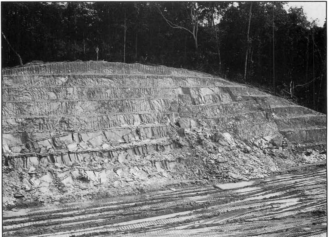
Figure 4. CH9300R. Major failure on right side of the slope involving 6 benches — planar failure along beddings. Note contrasting colours between grade IV (lower, grey) and grade V (upper, red/purple/orange/yellow) materials.
