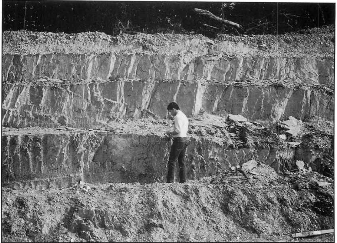
Figure 3. CH2300R. Grey shale with beds subparallel to the bench face. Prone to planar and/or toppling failure. Note hardly any residual soils over the shale.
