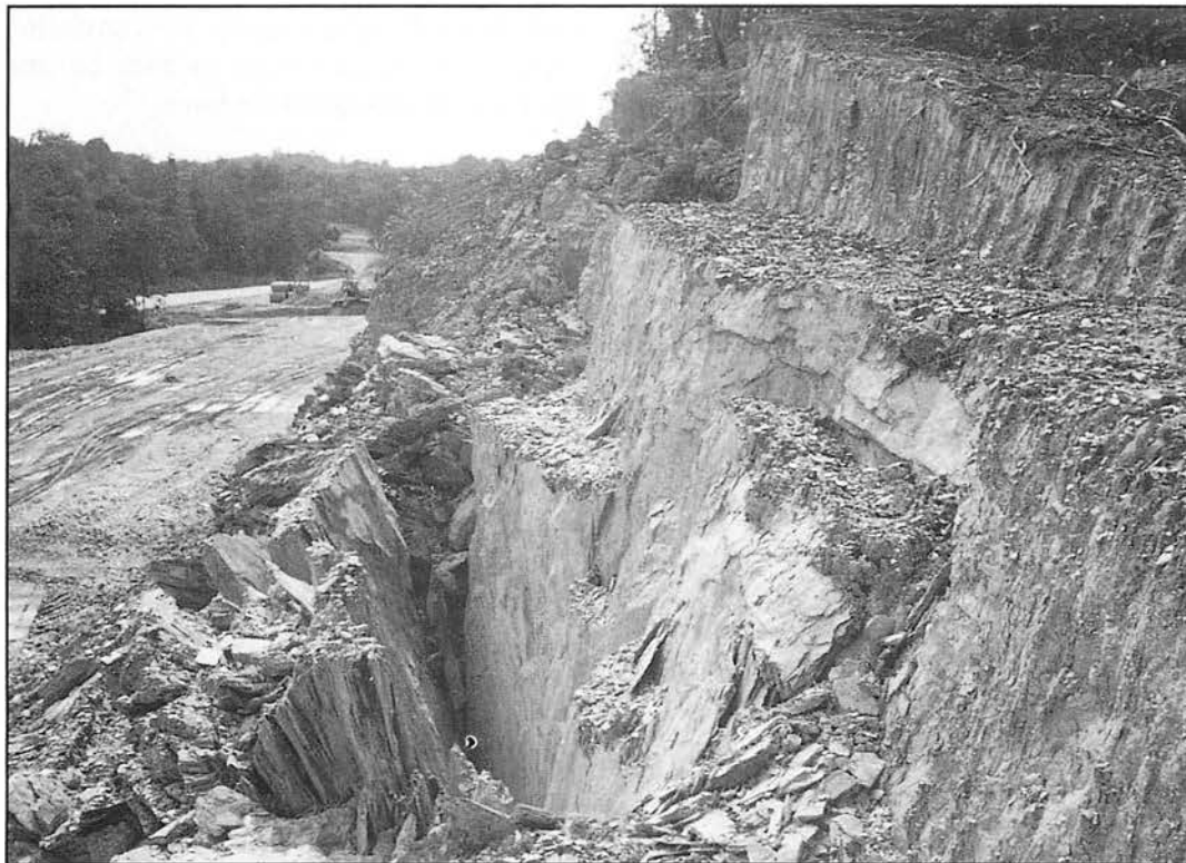
Figure 6. CH9300L. Toppling and opening up of tension cracks along beddings. Note parallelism of slope with bedding planes.
