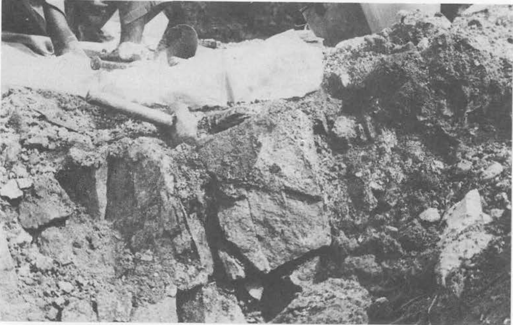
Plate 1. Mineralized vein and country rock broken up by blasting. Workers dislodged cassiterite-bearing rock using picks and hammers.
